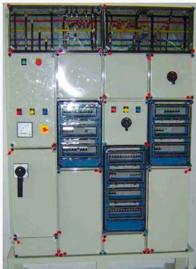
Main power distribution board for a petrol station
