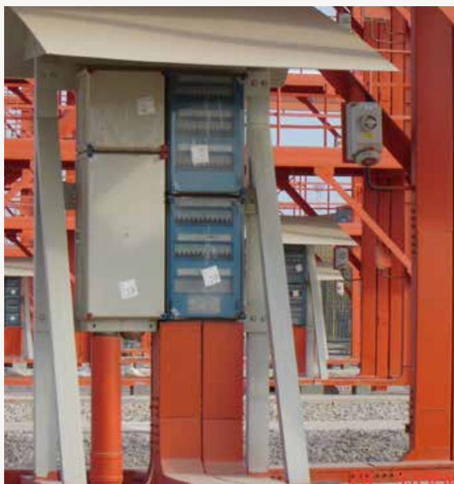
High mast lighting distribution board at a container yard
