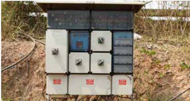
Sub distribution board installed at a hydro electric plant.
