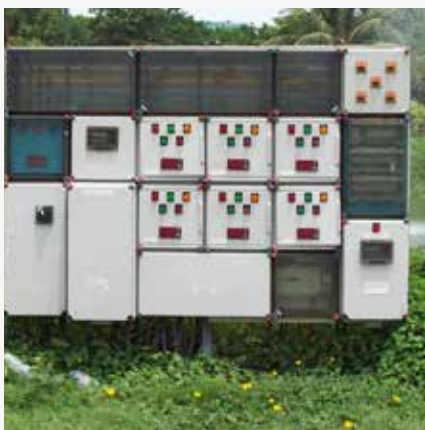
+ Outdoor distribution board installed at the lawns of a luxury hotel.
