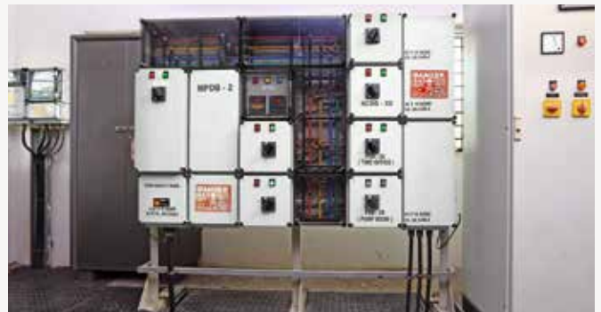
Main power distribution board installed at a foundry
