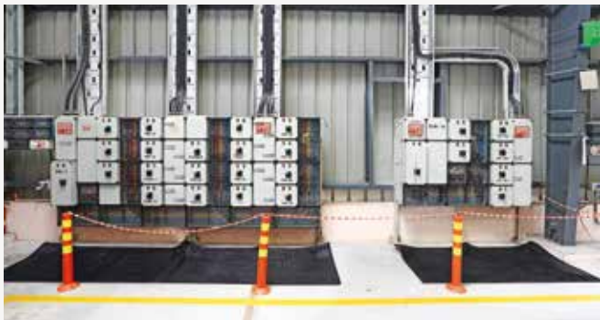
Power distribution boards installed at a light engineering industry
