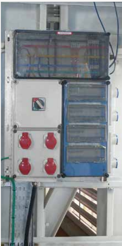
Shop floor distribution board with CEE sockets installed in an engineering fabrication plant.
