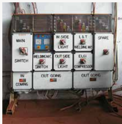
+ Power distribution board installed at a maintenance workshop of an iron ore mine
