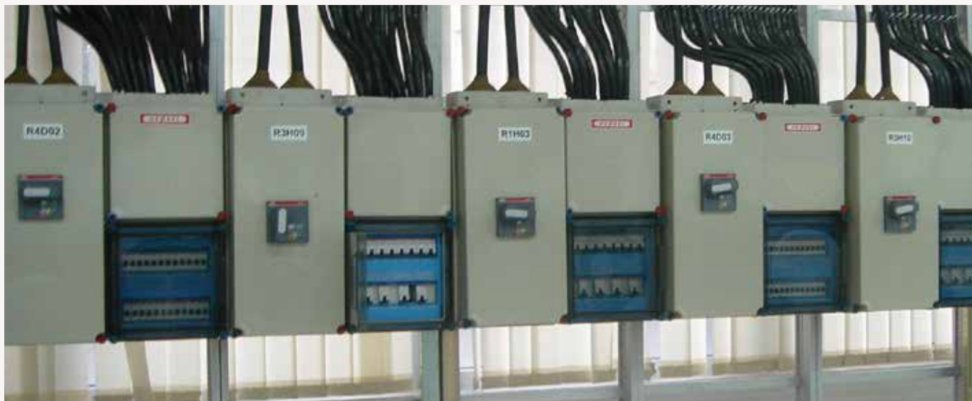
Lighting control distribution boards in use at a mobile phone manufacturing plant
