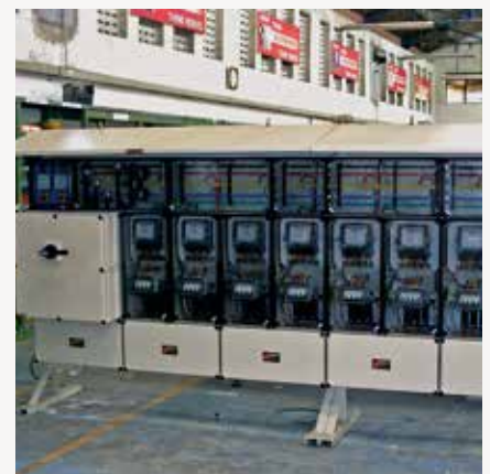
+ Metering panel with KWH meters for an electric supply utility company
