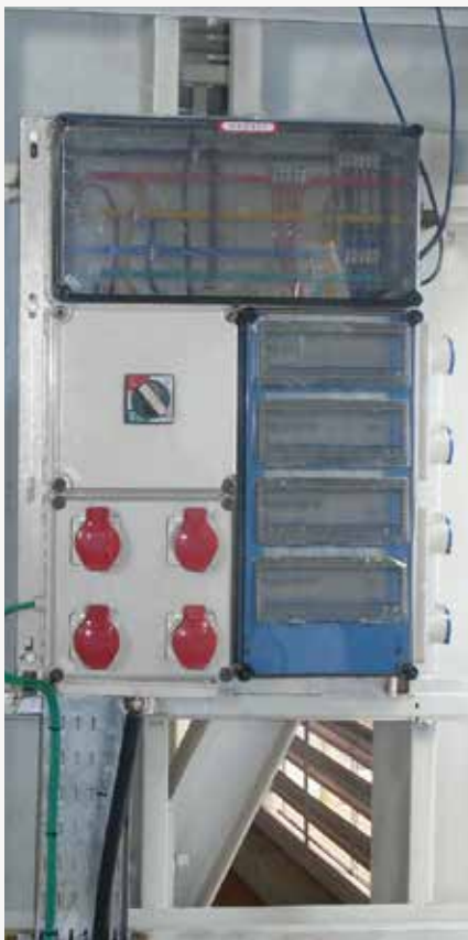
Shop floor distribution board with CEE sockets installed in an engineering fabrication plant.
