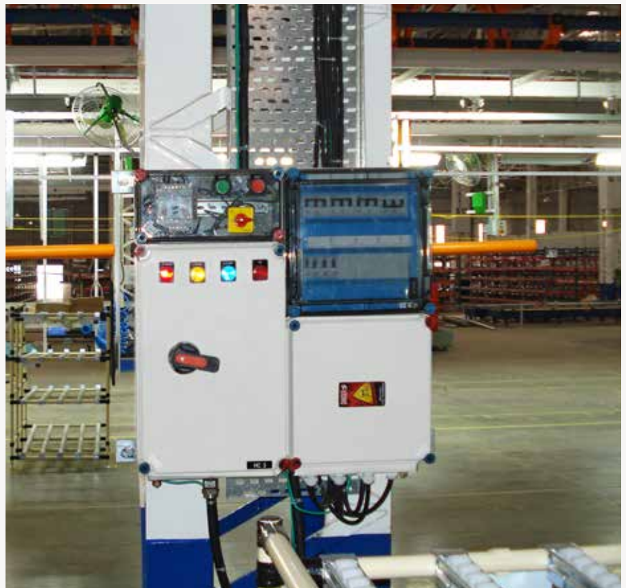
Lighting distribution board installed in body shop of an automobile plant.
