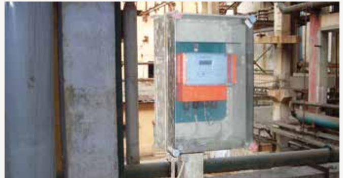
Instrument enclosure at a pumping station
