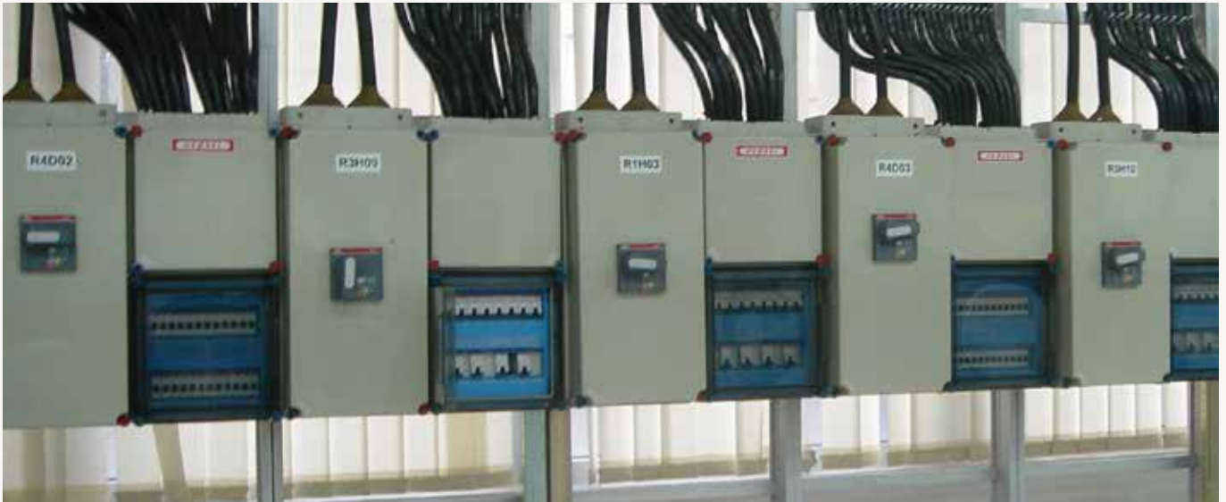
Lighting control distribution boards in use at a mobile phone manufacturing plant
