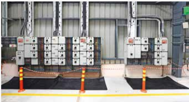
Power distribution boards installed at a light engineering industry
